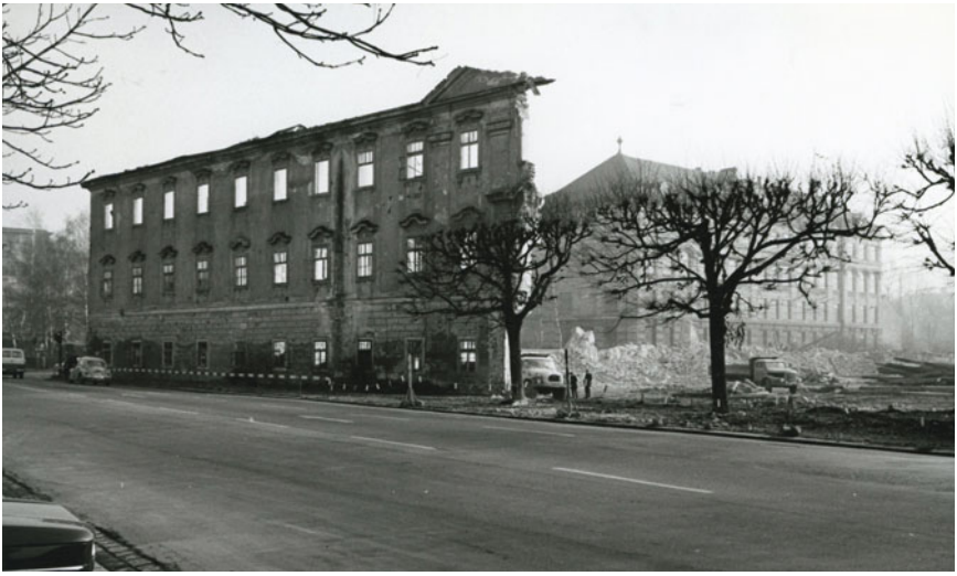
Demolition of the Wool Factory, 1969. Photo: Archives of the Nordico City Museum, Linz.
