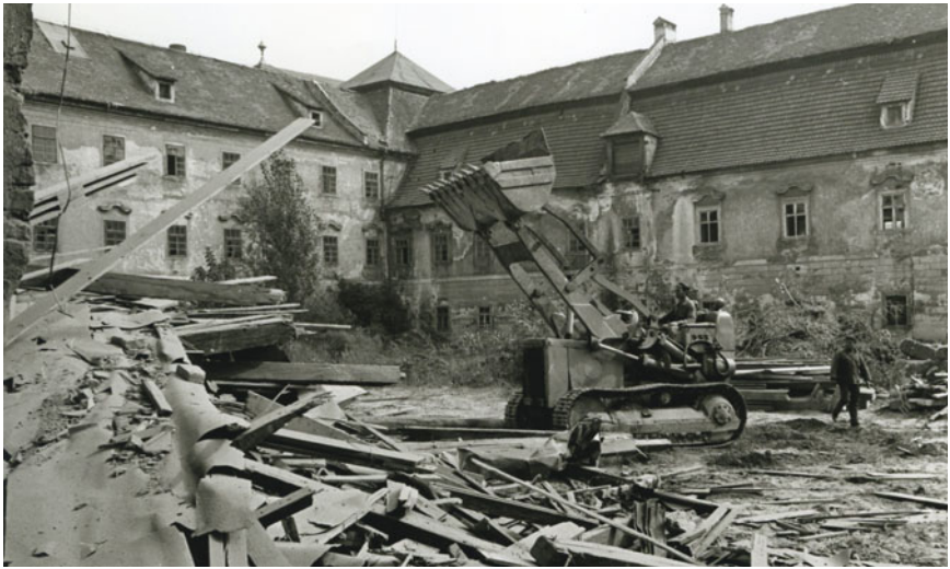
Demolition of the Wool Factory, 1969. Photo: Archives of the Nordico City Museum, Linz.
