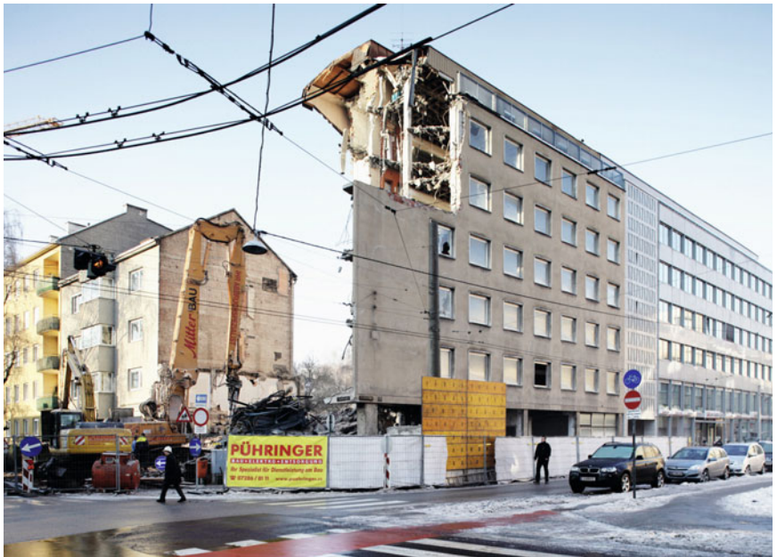
2010 demolition of the Community College, former Park Hotel, constructed in 1952 by Artur Perotti and Gottfried Zellingner. Photo: Gregor Graf.
